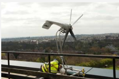
One of the nine turbines on the South Tower
